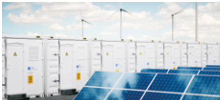
Battery energy storage systems (BESS)
